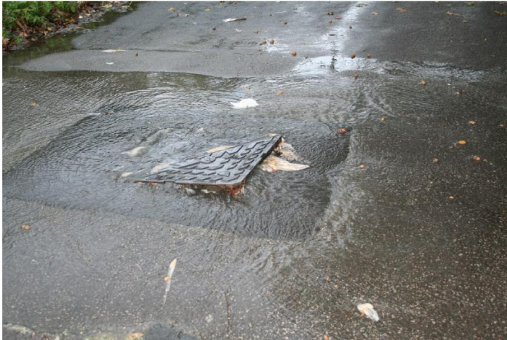
Image 12 – Sewage surcharge from manhole in Monkton Lane
